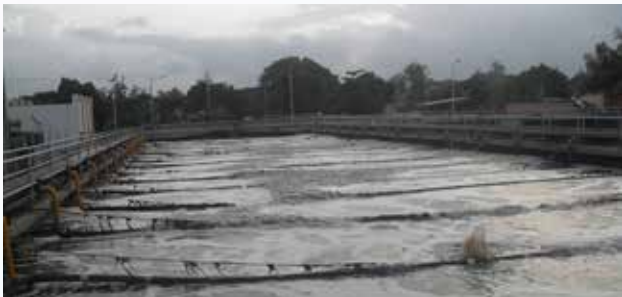
Common Effluent Treatment Plant
